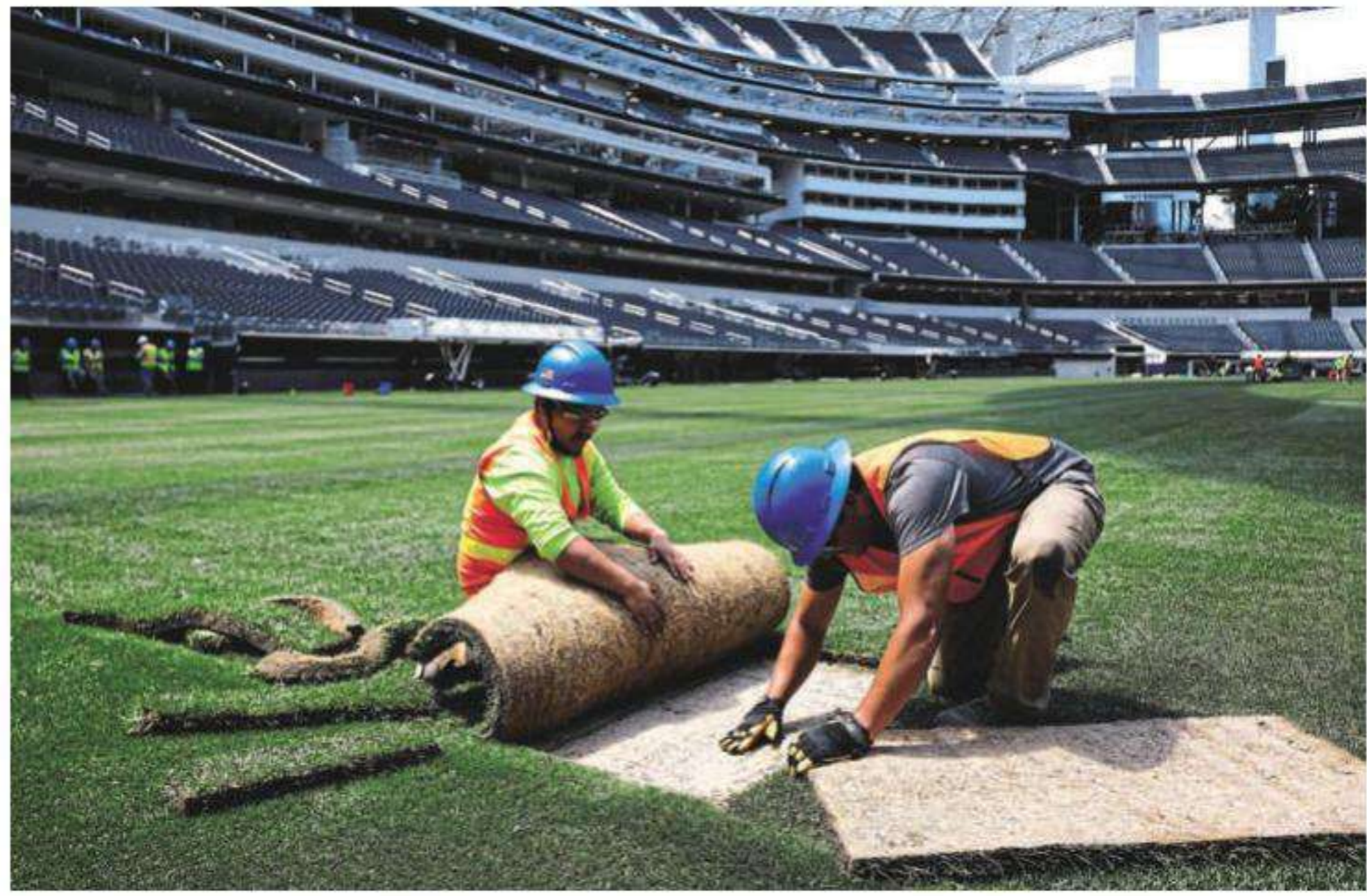
Workers, above and at right, install grass at SoFi Stadium in Inglewood, California, in May. For organizers and grass experts, each venue presented unique challenges.
